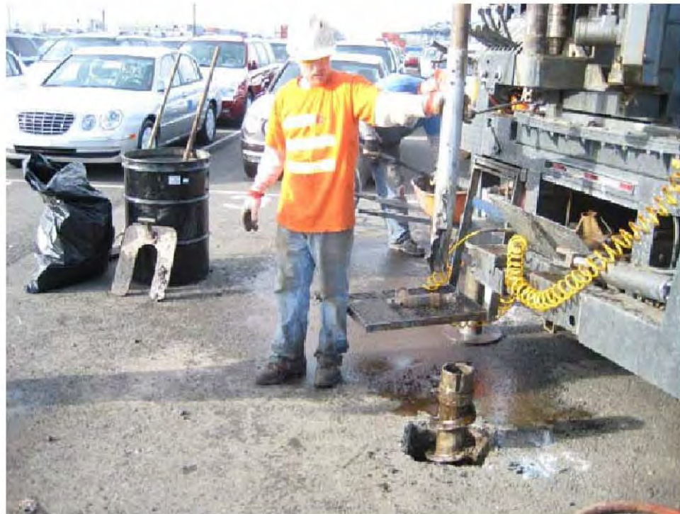
Photo 3. Core sampler damaged by subsurface rocks.
